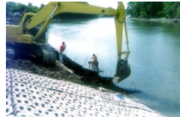
With backhoe, workers install specially designed concrete-block sections on the south bank of the Minnesota River in Burnsville — one of nine different experimental erosion-control methods the District is testing. Photo: Pete Willenbring.
